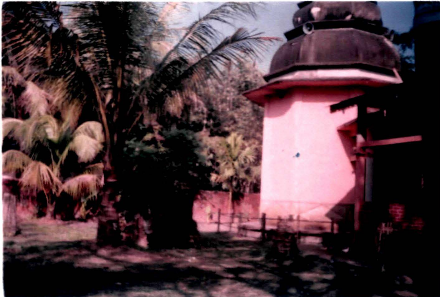
Plate 10 : Heavy sand deposition by Pagladiya river buried half an old temple (Below coconut tree)
