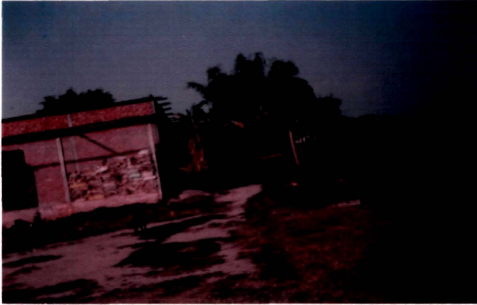
Plate 11 : Bank erosion collapsed the foundation of Pagladiya Dam Project site at Thalkuchi
