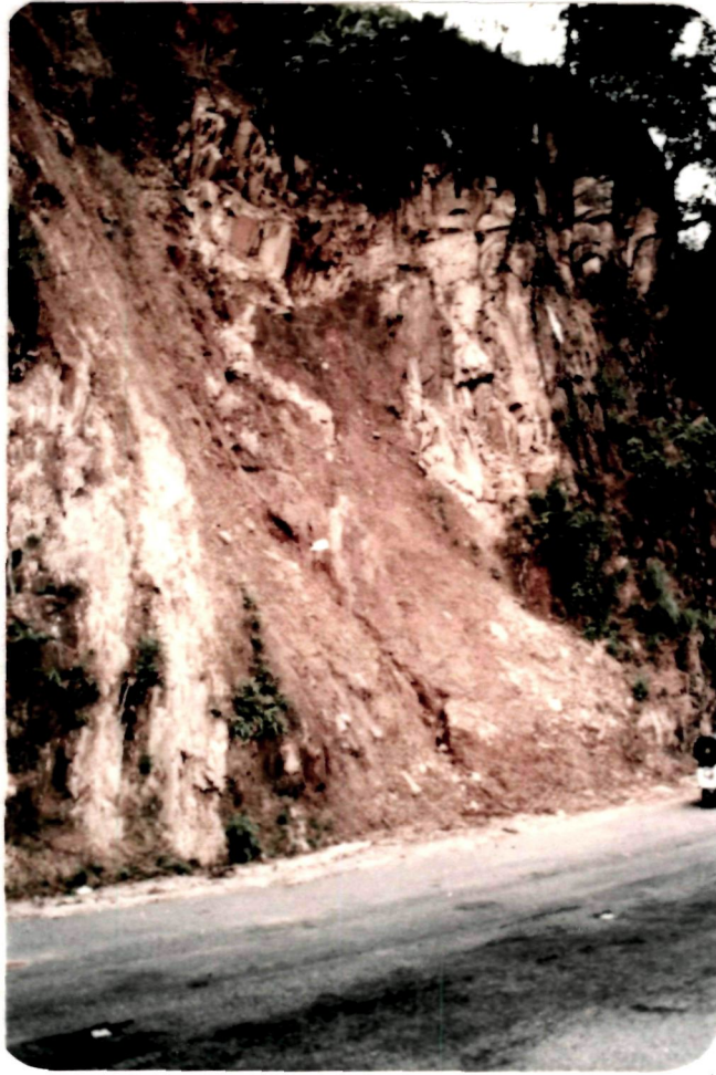
(Plate-6) : Initiation of physical weathering due to intersection of bedding/schistosity and subhorizontal joints (upper right corner) in quartzite.
