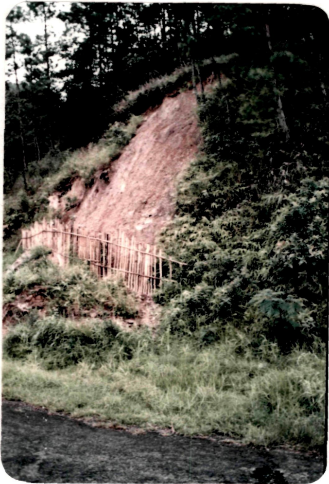
(Plate-9) : Landslide in sheared Phyllitic quartzite due to steep cuts on slope profiles. Note bamboo fence improvi- sation for temporary protection.
