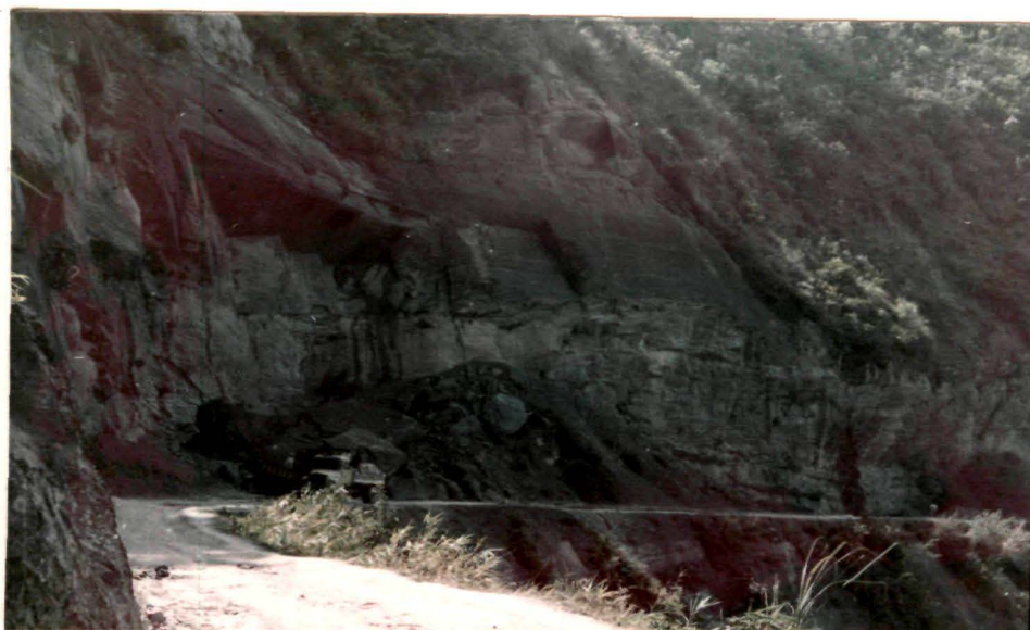
PLATE NO.3.8 :: Nature of terrain in Mizoram is a great hindrance to development of roads. The plate shows a State Highway under construction to connect Lunglei with Aizawl at a shorter distance .
