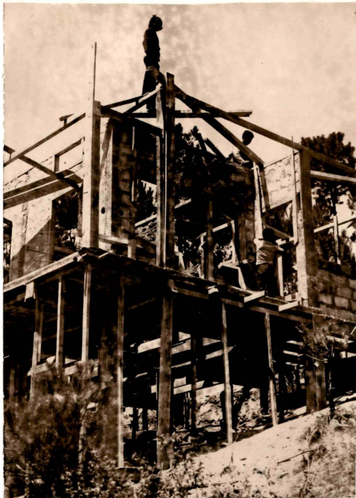
A hill slope settlement(Assam type) under construction. Note the length of the pillars
