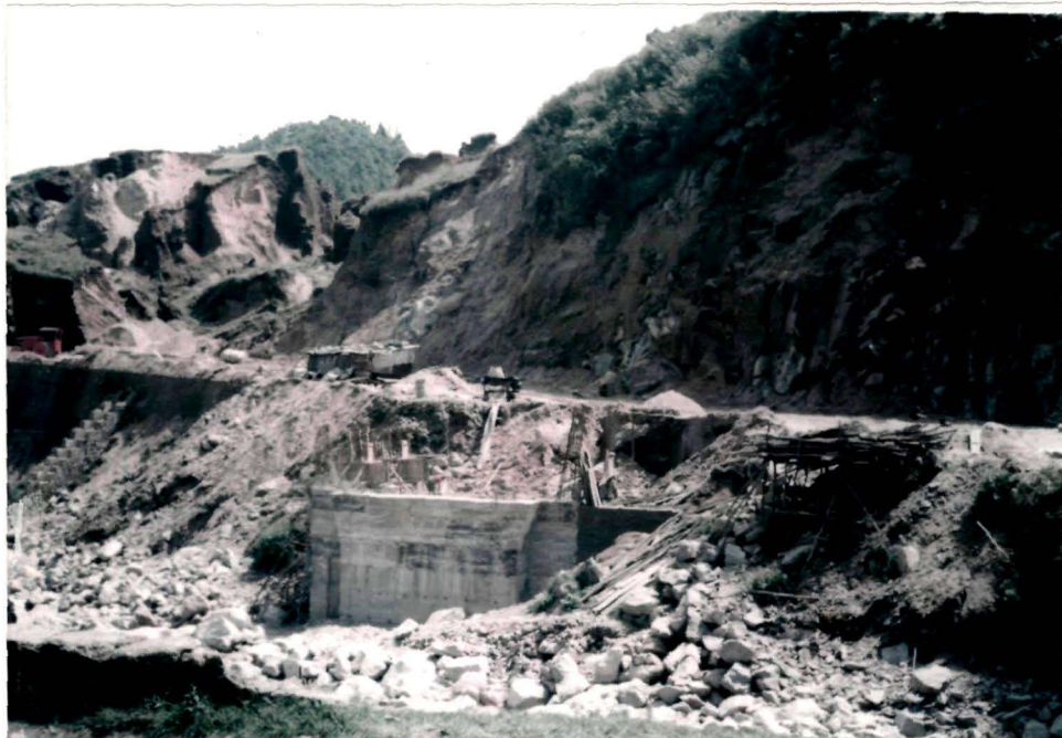
Plate 20a Blasting of rocks for road construction causing instability of hill slopes.
