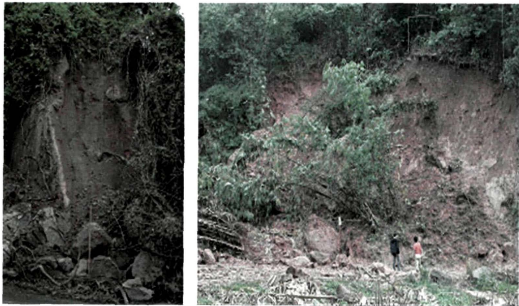
Figure 7.2: Debris fall and slumping
