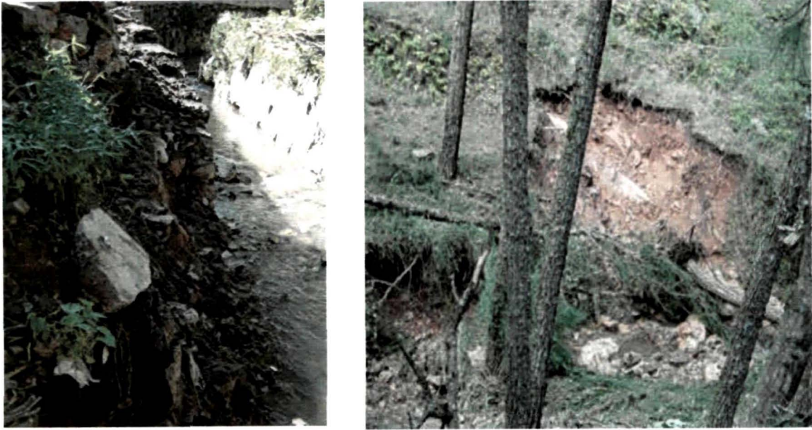
Figure 7.8: a. Breakage of the retention wall by the stream side during flash flood b. Debris fall near the stream at 4 th mile, Upper Shillong.
