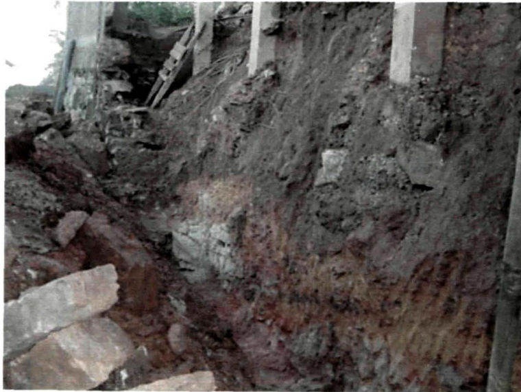
Figure 7.6: Breakage of the retaining wall in umlynka after heavy incessant rainfall where three people died on the spot.
