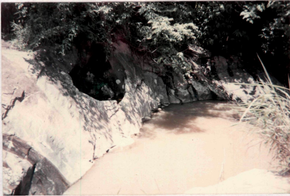
Plate 3(c): Eroded gneissic bed just above the drop.
