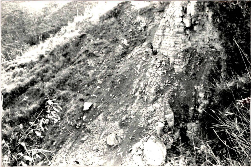
Surface Landslide on the steep slopes of loose sedimentary rock formation near Thingfal village
