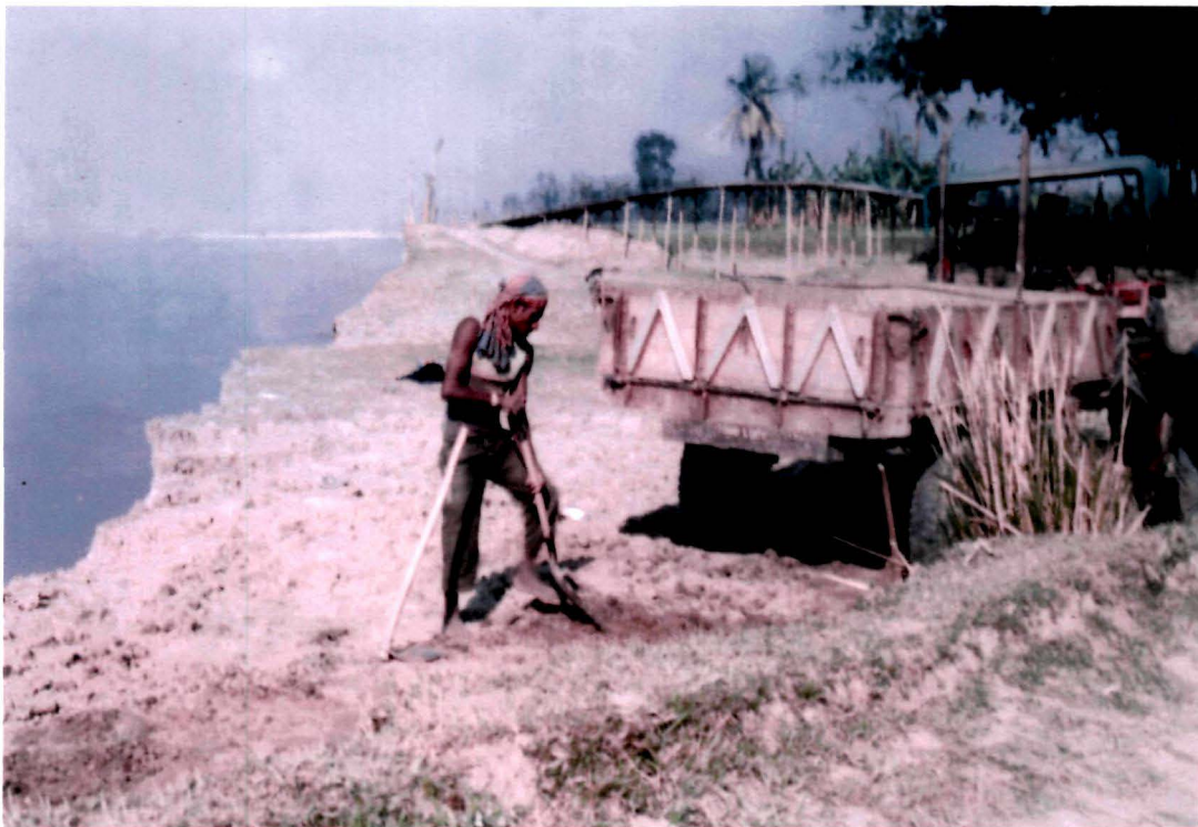
EARTH CUTTING NEAR RIVER BANK CONTRIBUTING TO EROSION
