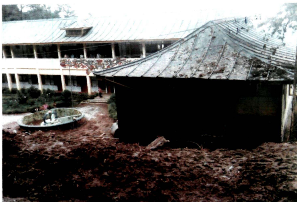
Plate 10 Debris of landslide filled compound of a government office near Zero Point
