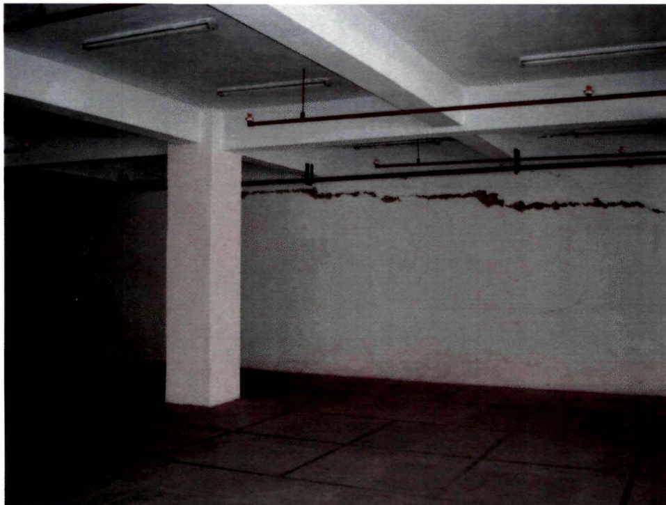
Plate 6 Cracks developed in a RCC building after the tremor of 5.7 intensity on 14.02.06
