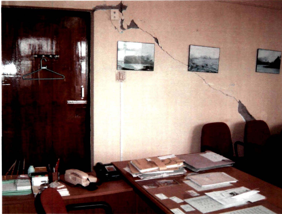
Plate 5 Cracks developed in a RCC building after the tremor of 5.7 intensity on 14.02.06
