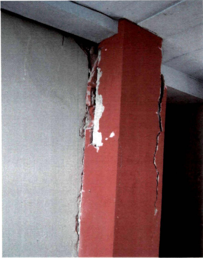
Plate 7 Cracks developed in a RCC building after the tremor of 5.7 intensity on 14.02.06
