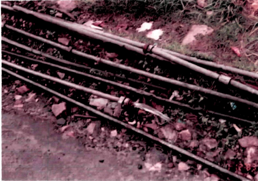
Plate 6.8 Leaking water pipes on the road side.
