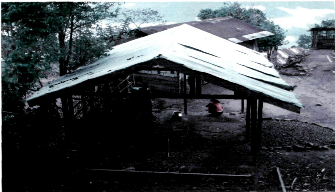
Plate- 14: Defunct Dispensary, Parbung village
