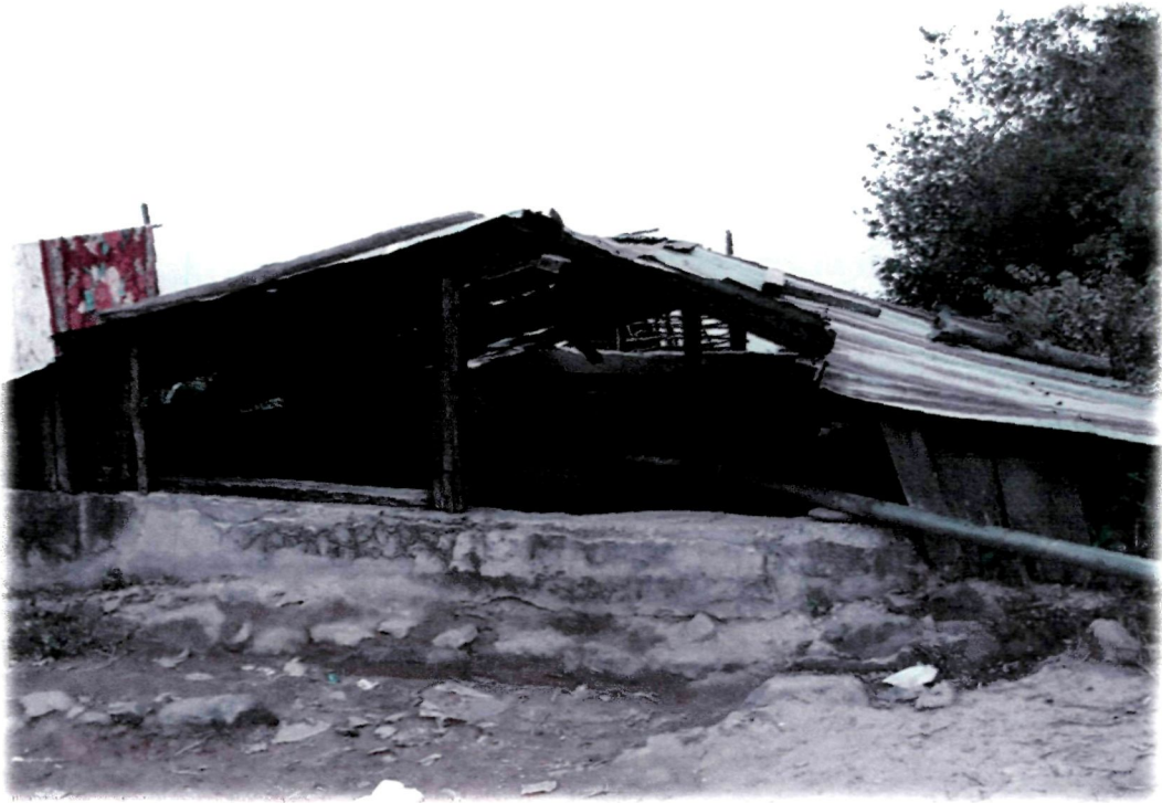
Plate- 15: Defunct water storage tank, Parbung village
